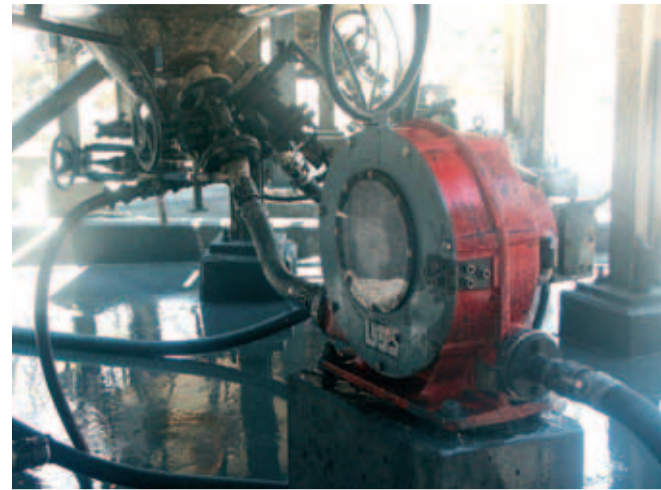
LPP-T in thickener underflow process
